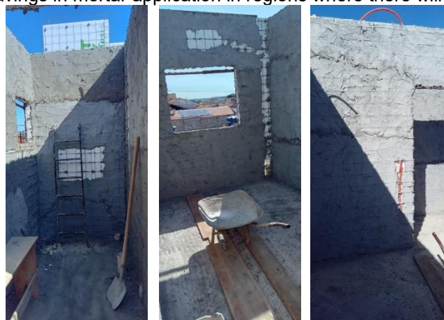
Figure 32 Savings in mortar application in regions where there will be no coating
