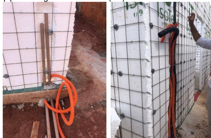
Figure 24 Passage of pipes through the foundation (left) and arrival of conduits in the EPS panel (right)
