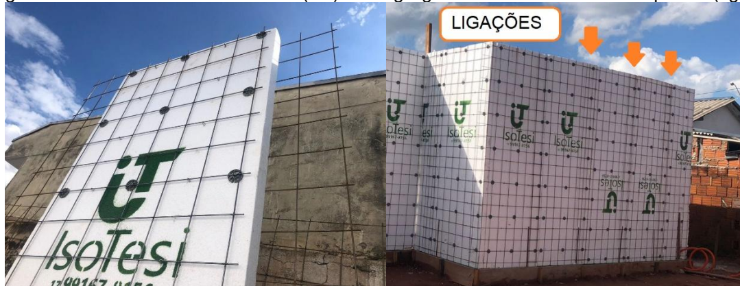
Figure 23 Extension of the steel mesh (left) and highlight for the connection of the panels (right)
