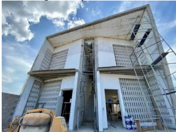
Figure 5 Construction using the ICF system carried out in the Northeast of Brazil
