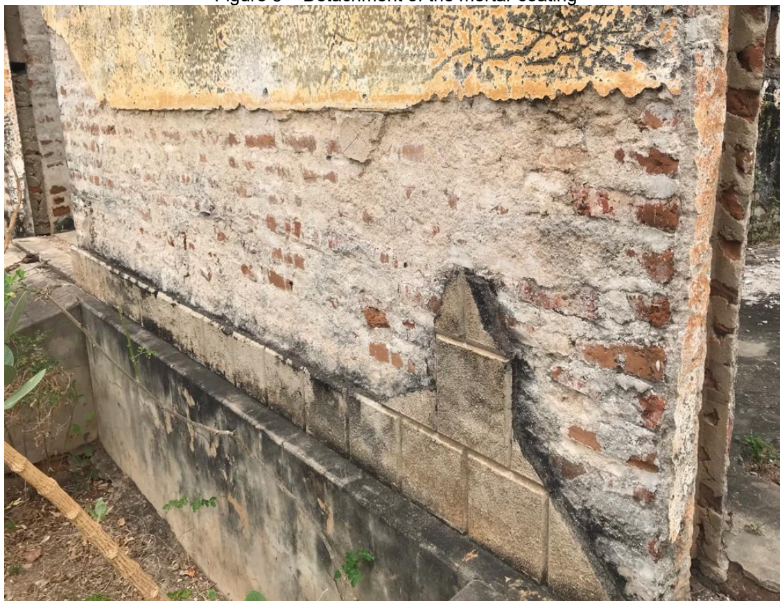
Figure 5 – Detachment of the mortar coating
